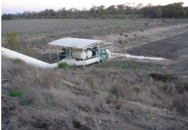
Pumping Station, transfers runoff from a drainage canal (ditch) to a ring tank for storage.
